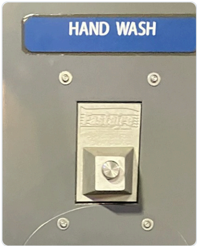
INSTALLED ABOVE THE PUSHBUTTON
