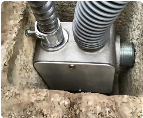
SWITCH BOX IN THE WALL Air hose and conduit run up from the switch box to the blower.
